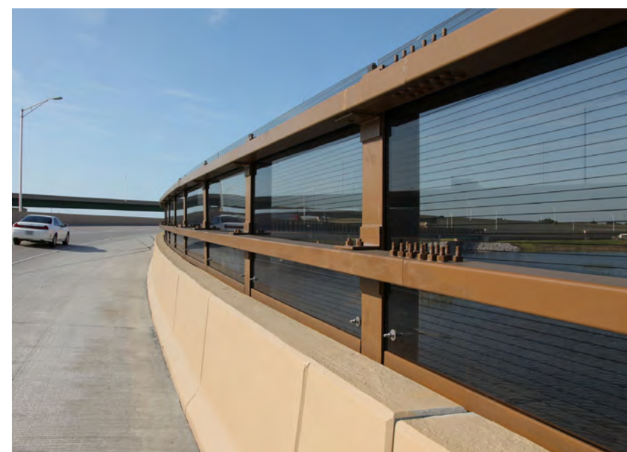
TRANSPARENT NOISE WALL - MOUNTED BEHIND BARRIER
